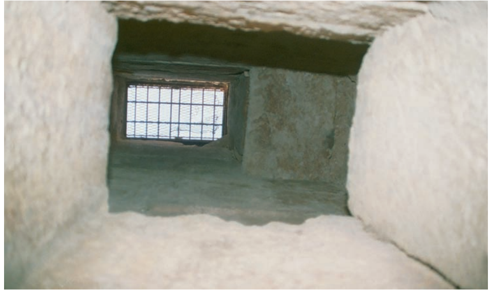
An opening in the ceiling
