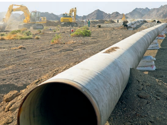
New water pipe
